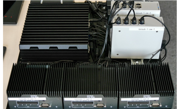
Figure 1. Photograph of the TSN testbed showing the three endpoints up-1 to up-3, the two switches sw-1 and sw-2, and the controller ctrl.
